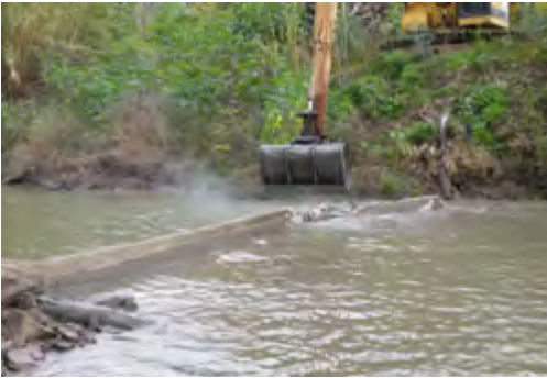
Removing or modifying old, redundant or unsafe weirs and culverts will all help our native fish recover. Photograph: Shona Whitfield.
